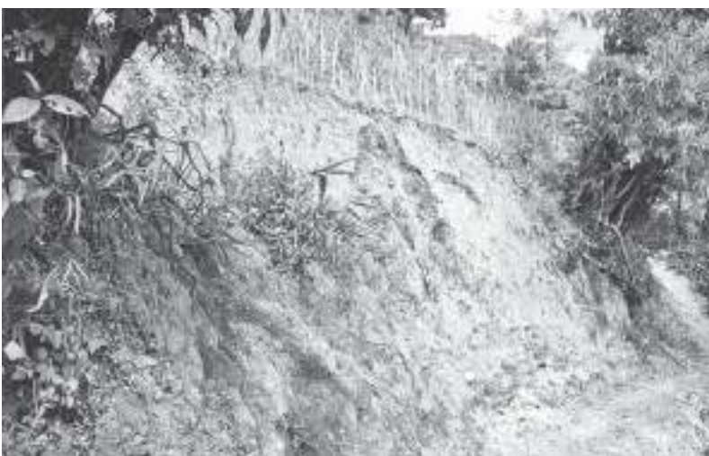
Picture 2.6a: Failed terrace edge, Dalchoki, Lalitpur (1993)
