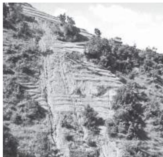
Picture 2.6b: Initiation of gullies from failed terrace edges, Dalchoki, Lalitpur (1992)
