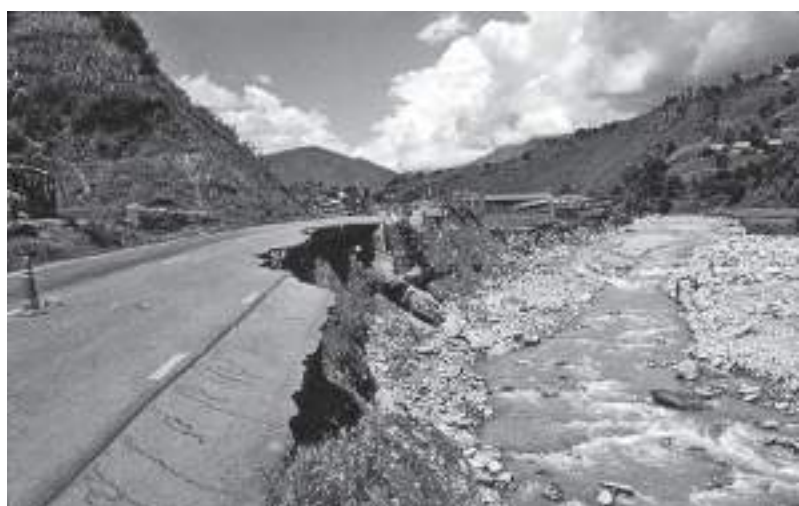
Picture 4.3: Damaged Prithivi Highway at Naubise, Dhading (1993)
