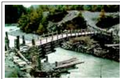
■ A new timber cantilever bridge on top of an old damaged one
